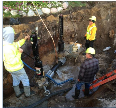
Construction crew installing line stops near the intersection of Monroe Blvd. and Streamwood Dr.
